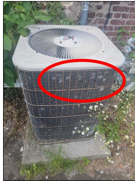
Damaged Condenser Fins Noted: Downstairs Unit
