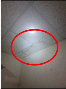
Drop Ceiling Tiles / Water Damaged: Downstairs Room 2
