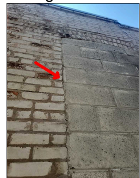
Cracks Noted In Mortar: Re-Point As Needed:
