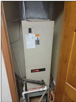
Upstairs Heater Location: Upstairs Apartment Heater Closet: Type: Electric
