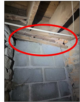
Wood Decay/Deterioration Noted: Basement
