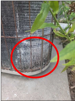
Damaged Condenser Fins Noted: Downstairs Unit
