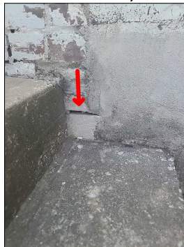
Missing Mortar Noted:
