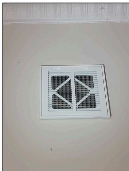
Filter Location: Downstairs Room 1
