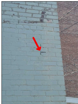
Missing Mortar Noted:
