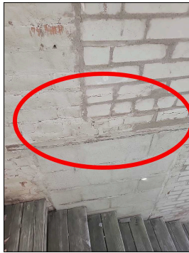
Cracks Noted In Mortar: Re-Point As Needed:
