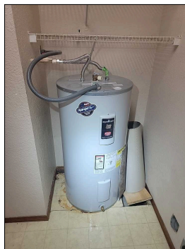
Water Heater Location: Apartment Bathroom; Type: Electric
