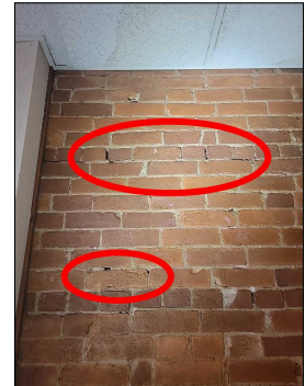
Failing Mortar: (Re-Pointing Advised): Upstairs Apartment
