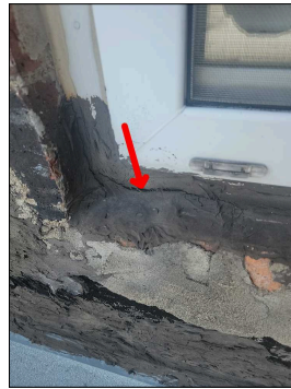
Cracked/Deteriorating Sealant Noted:
