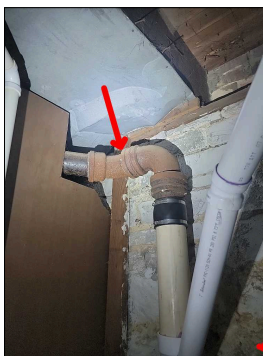
Cast Iron Lines Noted:
