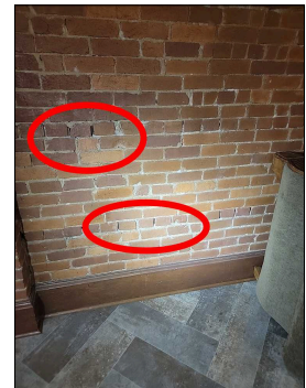
Failing Mortar: (Re-Pointing Advised): Upstairs Apartment
