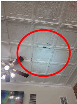
Previous Water Damage Noted: Downstairs Room 1
