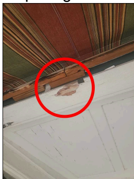
Peeling Paint Noted:
