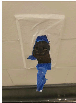
2-Prong (Ungrounded) Outlet: Downstairs Room 1
