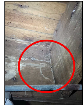
Termite Mud Tubes Noted: NW Corner
