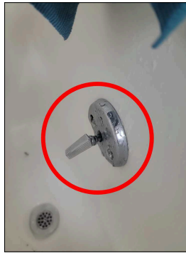
Stopper Missing/Inoperable: Apartment Bathroom
