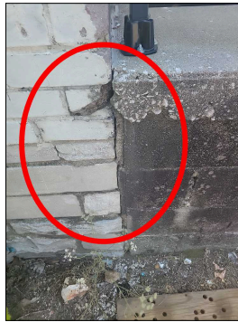
Failing Mortar: (Re-Pointing Advised):
