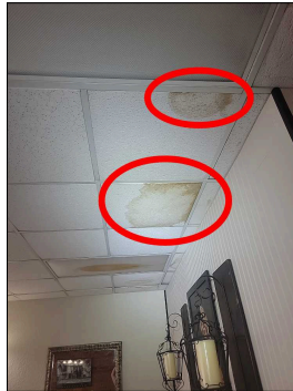
Drop Ceiling Tiles / Water Damaged: Downstairs Room 1
