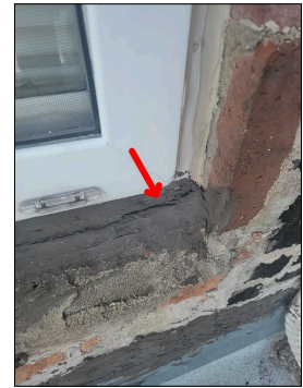
Cracked/Deteriorating Sealant Noted:
