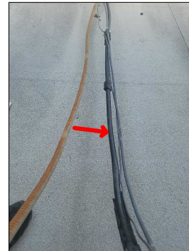
Line Set Insulation Old/Damaged/Missing: Upstairs Unit
