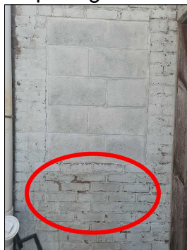
Failing Mortar: (Re-Pointing Advised):
