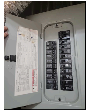
Unlabeled Breakers/Incomplete Or Missing Legend:
