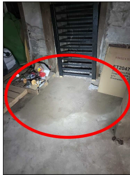
Signs Of Moisture Intrusion:
