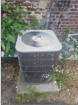
Downstairs A/C Location: W Side: Type: Electric
