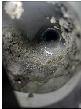
Dirty/Full Of Lint (Fire Hazard):
