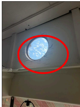
Water Damage Noted: Downstairs Room 1
