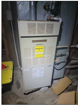
Downstairs Heater Location: Basement: Type: Electric Forced Hot Air
