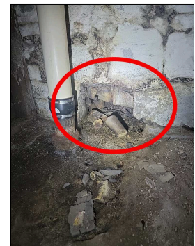
Loose/Missing Stones Noted:
