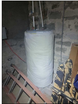
Water Heater Location: Basement; Type: Electric
