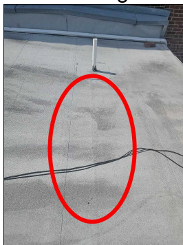
Wrinkles Noted In Rolled Roofing:
