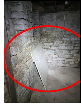
Moisture Intrusion Through Foundation:
