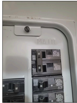
Main Amp Capacity: 100 Amp
