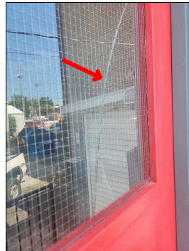
Cracked/Broken Glass: West Entry
