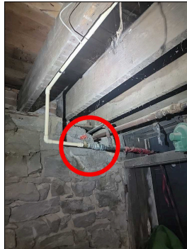
Main Shut Off Valve: Basement
