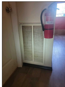
Filter Location: Downstairs Hallway
