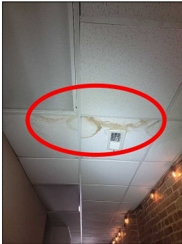
Drop Ceiling Tiles / Water Damaged: Downstairs Room 1
