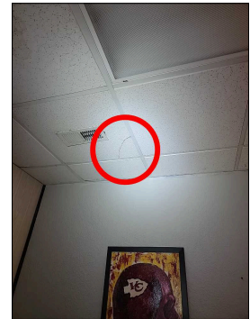
Damaged Ceiling Tile Noted: Downstairs Room 2
