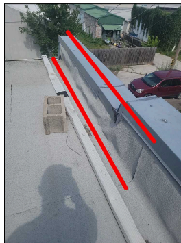
Wrinkles Noted In Rolled Roofing:
