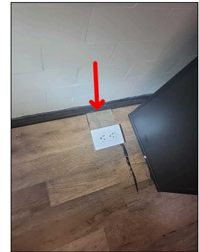
Improper Repairs Noted: Downstairs Room 1
