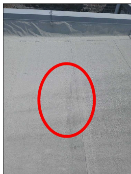
Soft Decking/Sheathing Noted:
