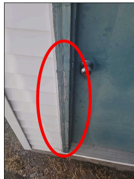
Peeling Paint Noted On Door Trim: West Entry
