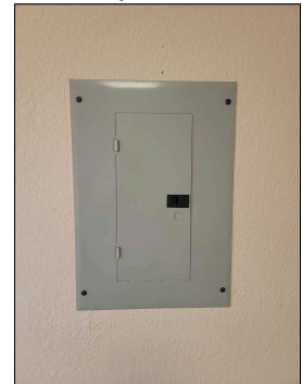
Main Panel Location: Apartment Bedroom
