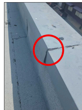
Sealant Wearing Out: Add Sealant:
