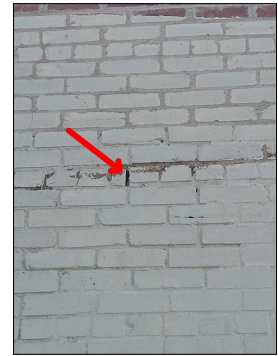
Missing Mortar Noted:
