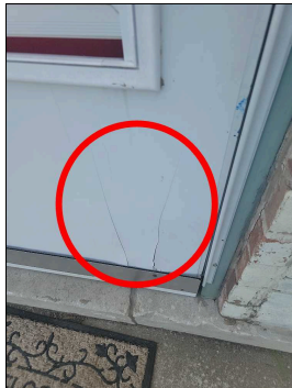
Cracks Noted In Screen Door: West Entry
