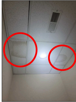
Drop Ceiling Tiles / Water Damaged: Downstairs Bathroom
