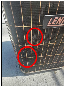
Damaged Condenser Fins Noted: Upstairs Unit
