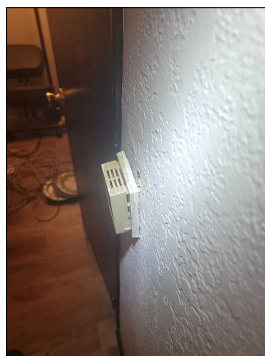
Loose Thermostat Noted: Downstairs Room 2
