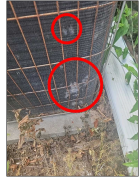
Damaged Condenser Fins Noted: Downstairs Unit
