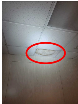
Drop Ceiling Tiles / Water Damaged: Downstairs Room 2
