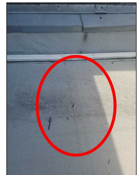
Wrinkles Noted In Rolled Roofing:
