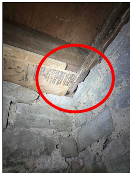
Signs Of Termite Damage: NW Corner
