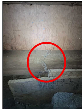
Termite Mud Tubes Noted: NW Corner
