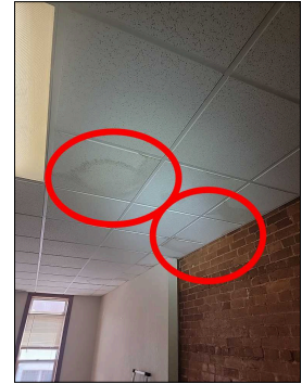
Drop Ceiling Tiles / Water Damaged: Upstairs Apartment Kitchen
