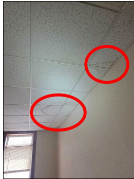
Drop Ceiling Tiles / Water Damaged: Upstairs Apartment Living Room
