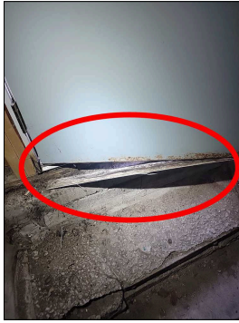
Loose Damaged Track On Bottom Of Door: Basement Entry
