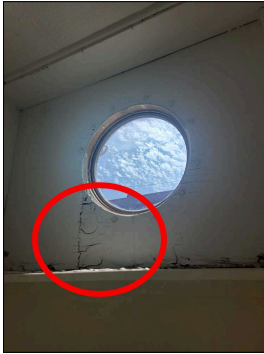
Water Damage Noted: Downstairs Room 1
