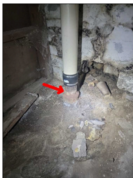
Cast Iron Lines Noted:
