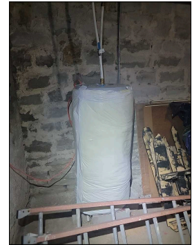
Insulation Blanket - Water Heater Casing Not Visible Due To Insulation Blanket: Downstairs Unit
