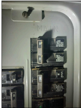
Main Amp Capacity: 100 Amp
