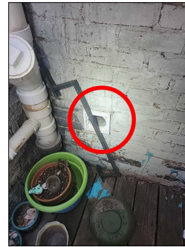
Dryer Vent Cover Missing:
