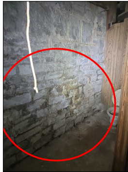
Moisture Intrusion Through Foundation:
