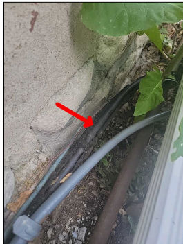
Line Set Insulation Old/Damaged/Missing: Downstairs Unit
