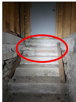
Cracked/Deteriorating Concrete Noted: Basement Steps To Outside
