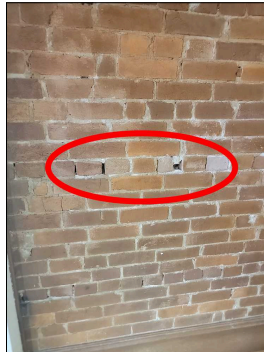
Failing Mortar: (Re-Pointing Advised): Upstairs Apartment
