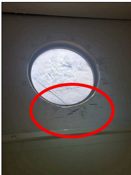
Water Damage Noted: Downstairs Room 1
