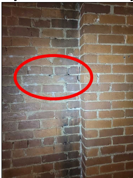
Failing Mortar: (Re-Pointing Advised): Upstairs Apartment
