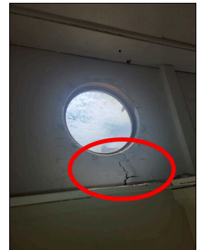
Water Damage Noted: Downstairs Room 1
