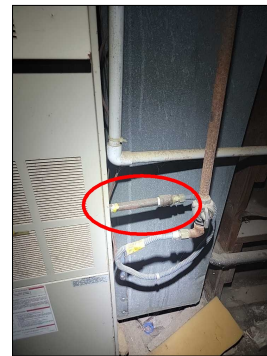
Gas Supply Line Missing Drip Leg:
