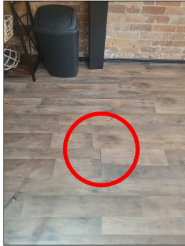
Soft Spot Under Flooring: Downstairs Room 1
