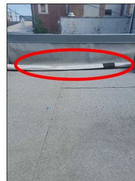
Downspout Crushed: Will Restrict Water Flow
