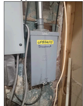
Breaker Location For Upstairs Unit:
