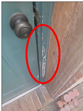
Peeling Paint Noted On Door Trim: Apartment Entry
