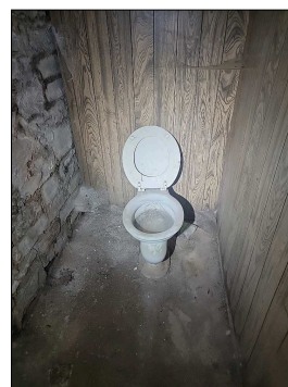
Toilet Inoperable: Basement
